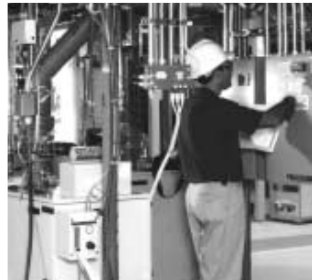
Pre-programmed controllers are available with alarms, remote communication packages and other custom features. (16 zone MLS controller shown)
